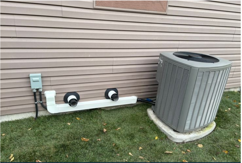
Outdoor condenser installation
