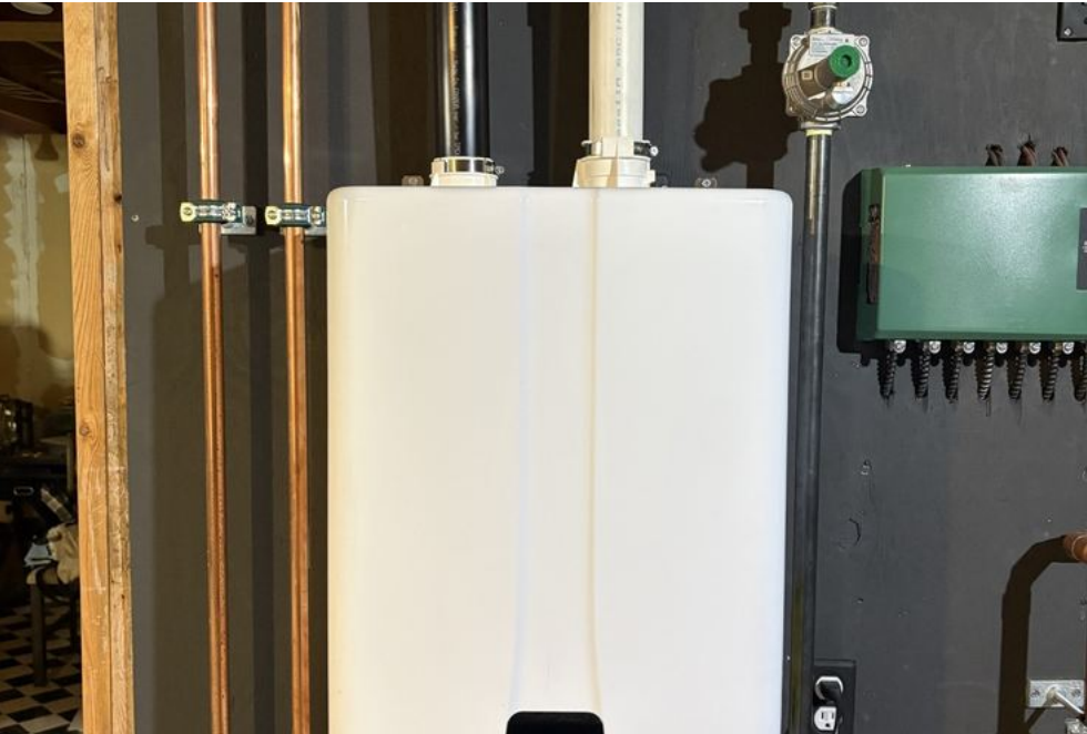
Navien tankless installation
