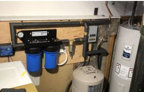
Water treatment equipment
