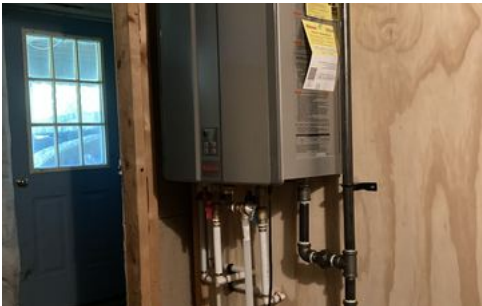
Water heating installation
