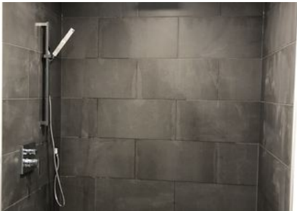
Shower plumbing and fixtures
